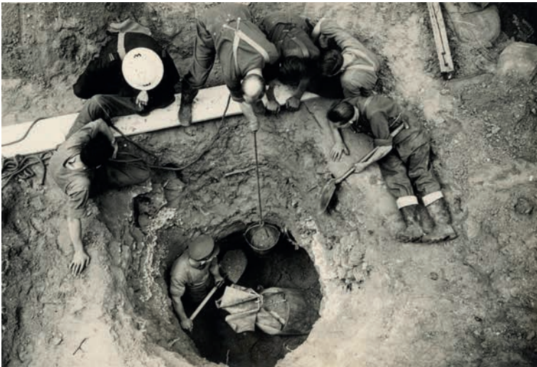
Working against time, Royal Engineers dig out an unexploded German 1,000kg bomb, half of which is still embedded at a depth of more than twenty feet, in the grounds of the German Hospital, Dalston, September 1940. All patients had been evacuated and there were no casualties. ( Historic Military Press )
